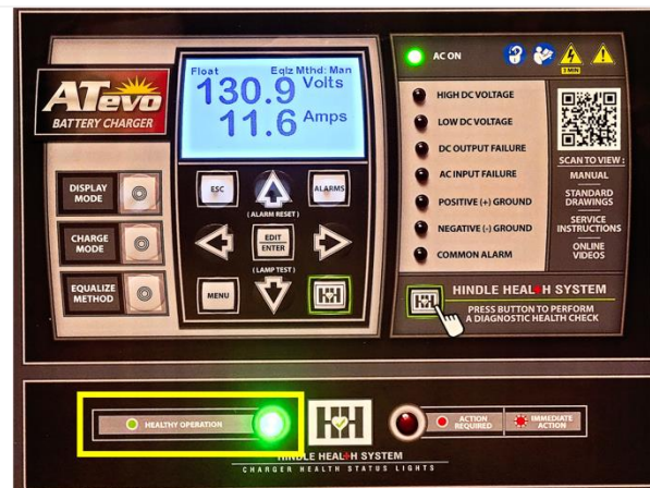
Figure 2A – Status LED for Healthy Operation
